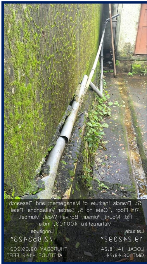
BMC Pipe Line
