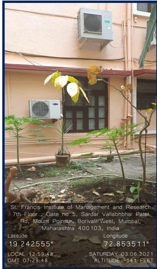
Brought down by vertical & Horizontal Pipes
