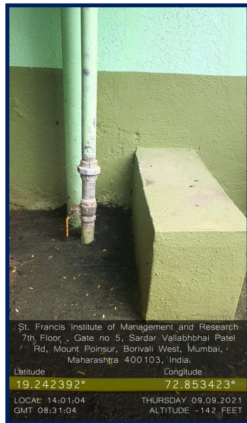
Pipeline from bore well tank to Hostel
