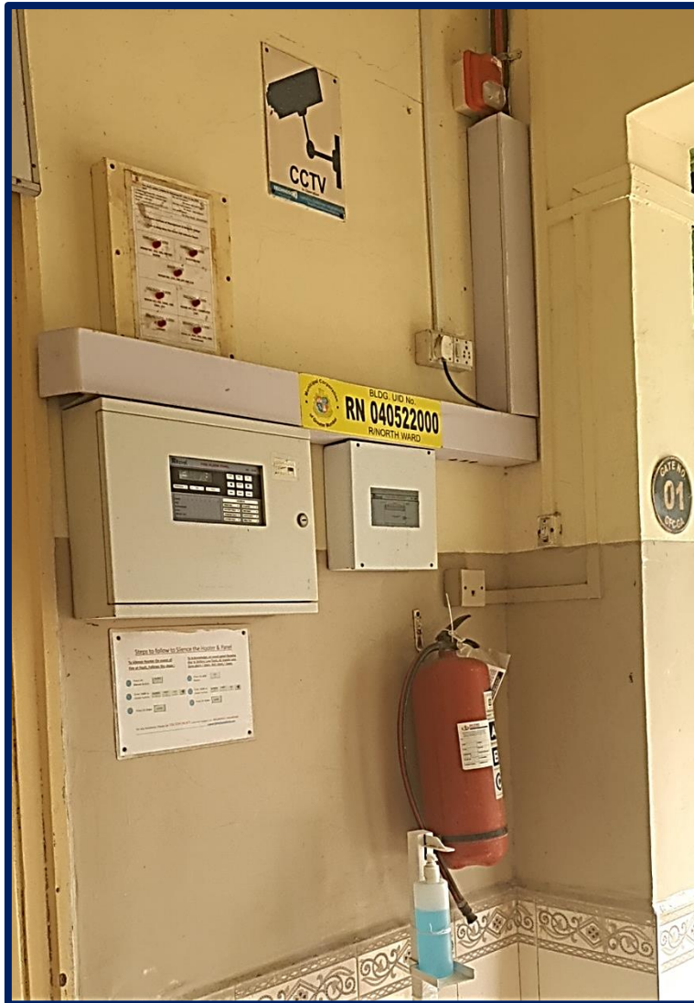
Fire Alarm, Fire Extinguisher and CCTV Surveillance in SFIMAR Campus
